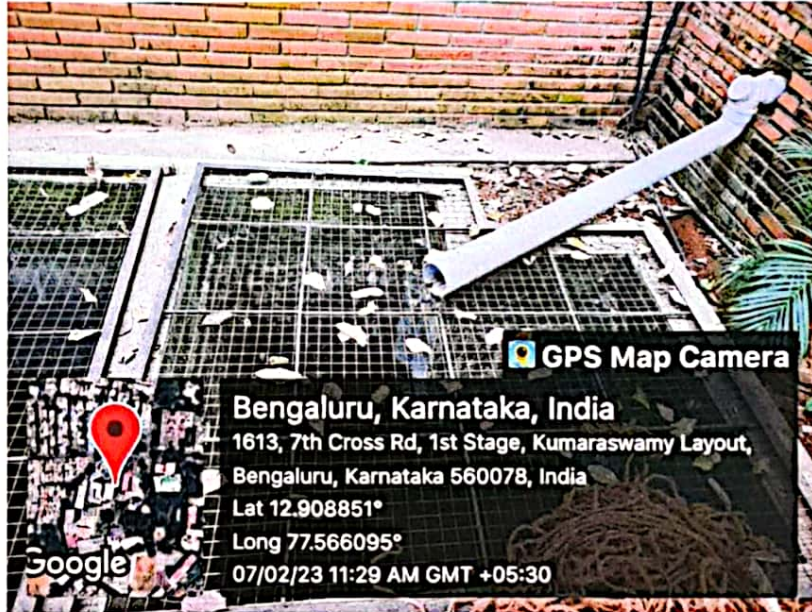
RAINWATER HARVESTING NEAR DSCDS FACILITIES DEPARTMENT
