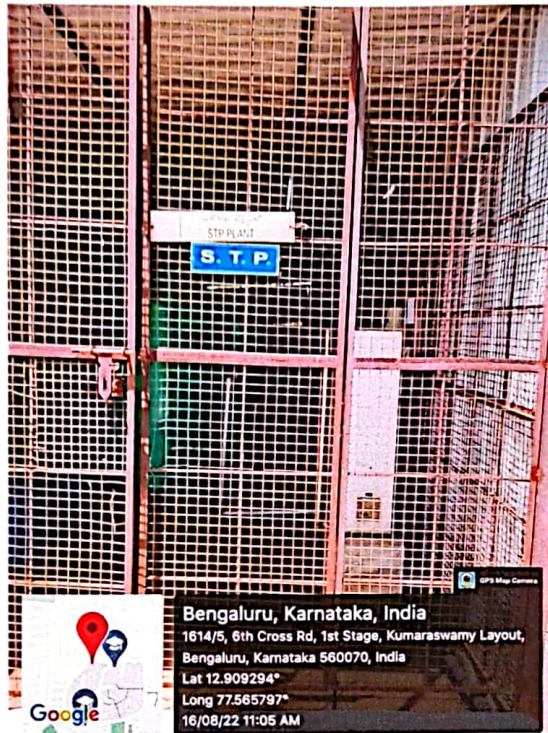
SEWAGE TREATMENT PLANT
